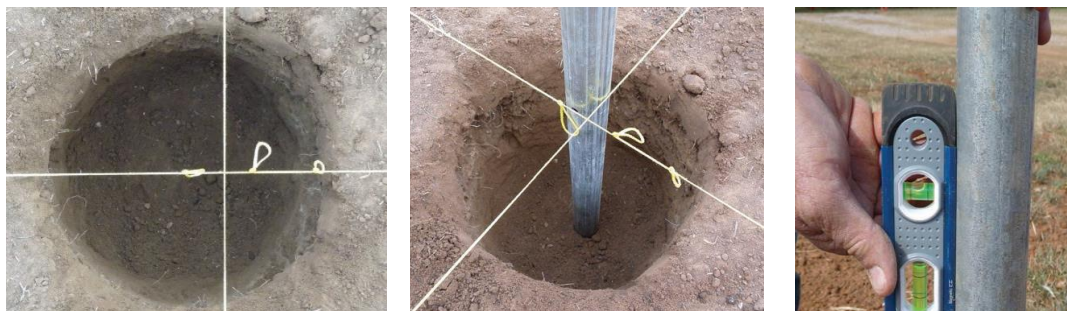
Figure 18: (a) Corner hole (b) Setting the foundation pipe in the corner holes (c) Checking level of the foundation pipe
