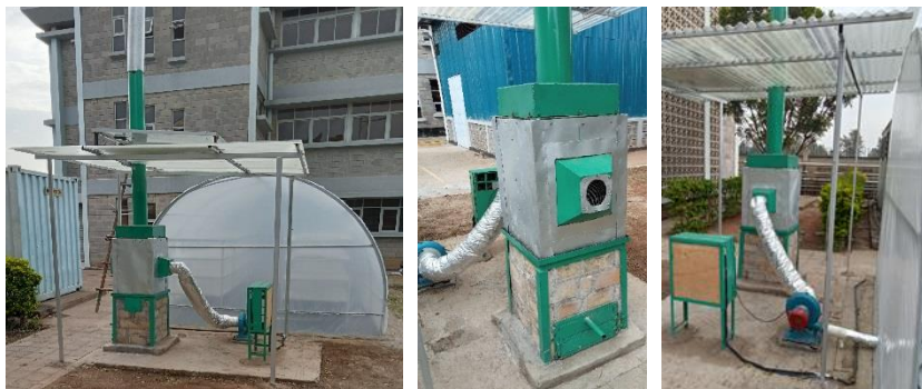
Figure 29: Connection of Biomass heat exchanger system with the hot air distribution ducting
